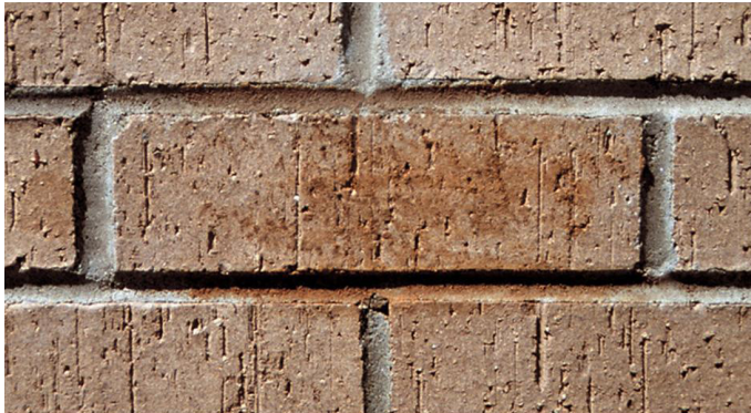
Photo 1: Manganese Stain on Brick
