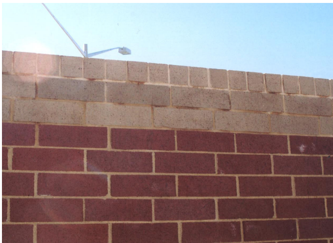
Photo 2: Manganese Stain in Mortar Joints
